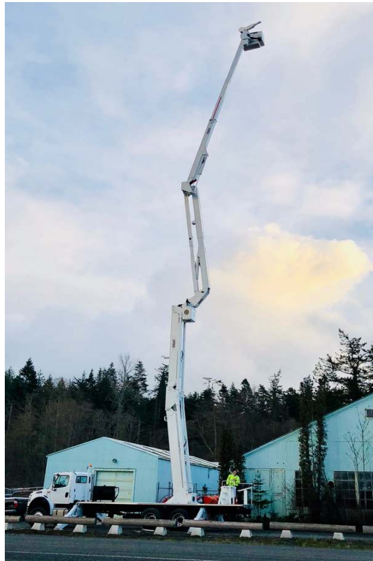
Meet "Ursula" our new 113' Bucket Truck for building and maintaining our LTE Sites
